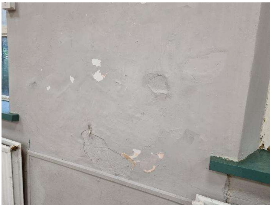
82. Damp and defective plaster noted
