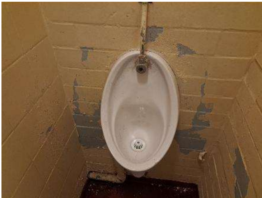
4. View of aged urinal and poor decoration
