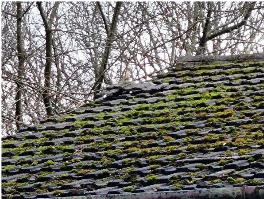
92. View of damaged Roof Tile
