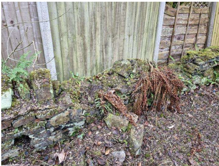
117. Boundary Wall is in poor condition
