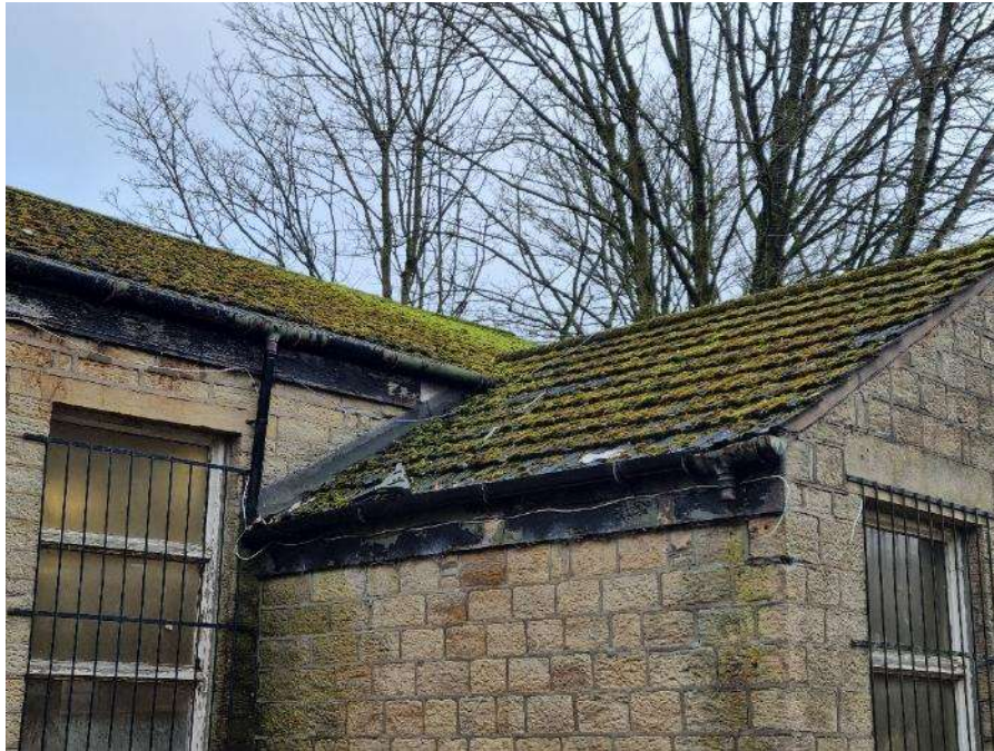
93. View of damaged roof
