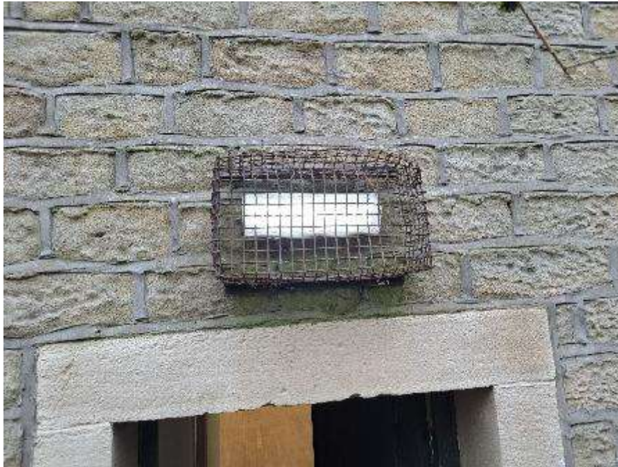
137.Damaged basket light guard
