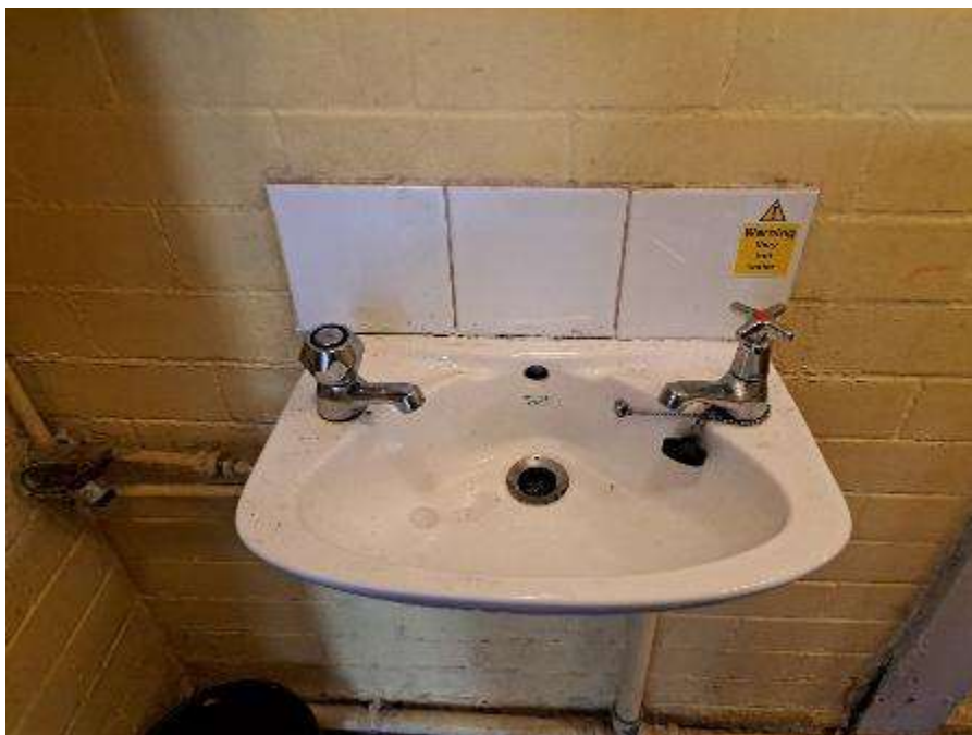
2. Sink and tiles in dirty and aged condition
