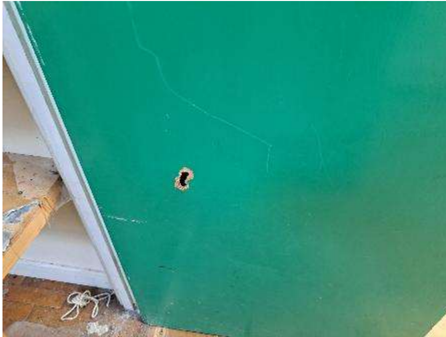
43. Impact damage to the door
