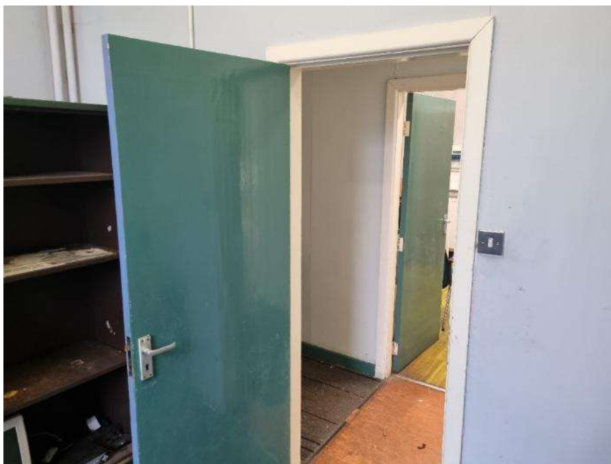
62. The door is in fair condition consider replacing.
