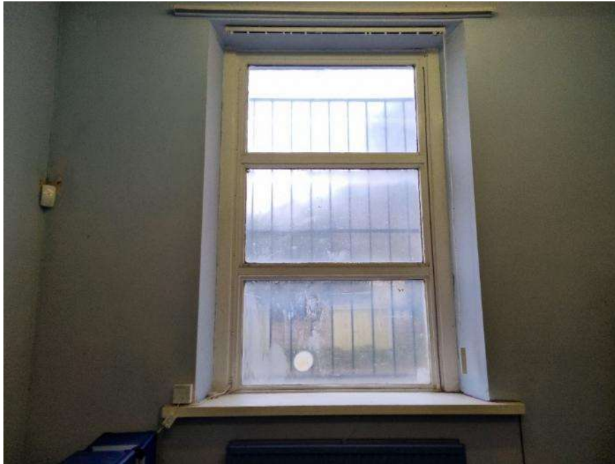
63. Window is in poor condition
