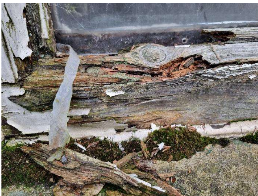
110. Window is in poor condition
