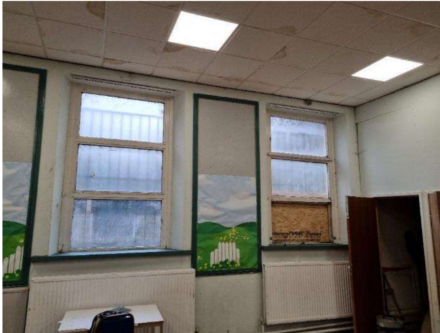
85. Windows are in poor condition
