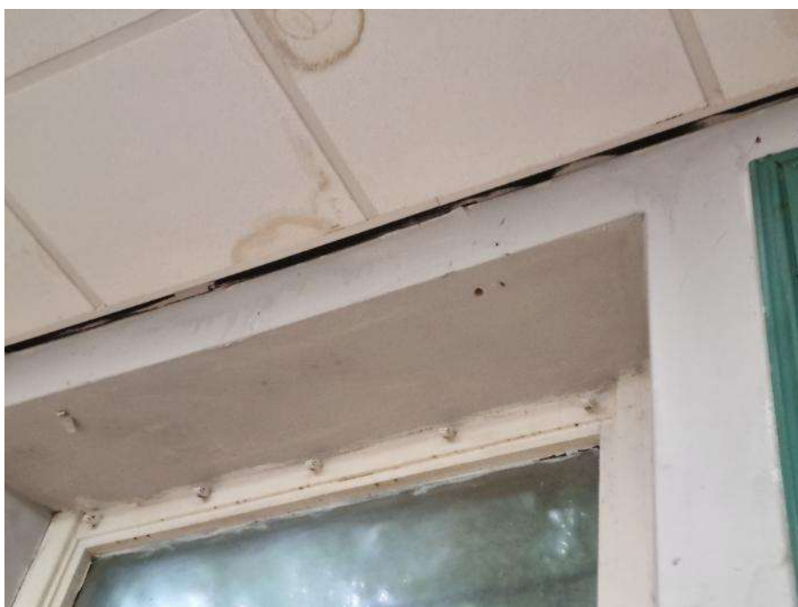
90. Ceiling is in poor condition
