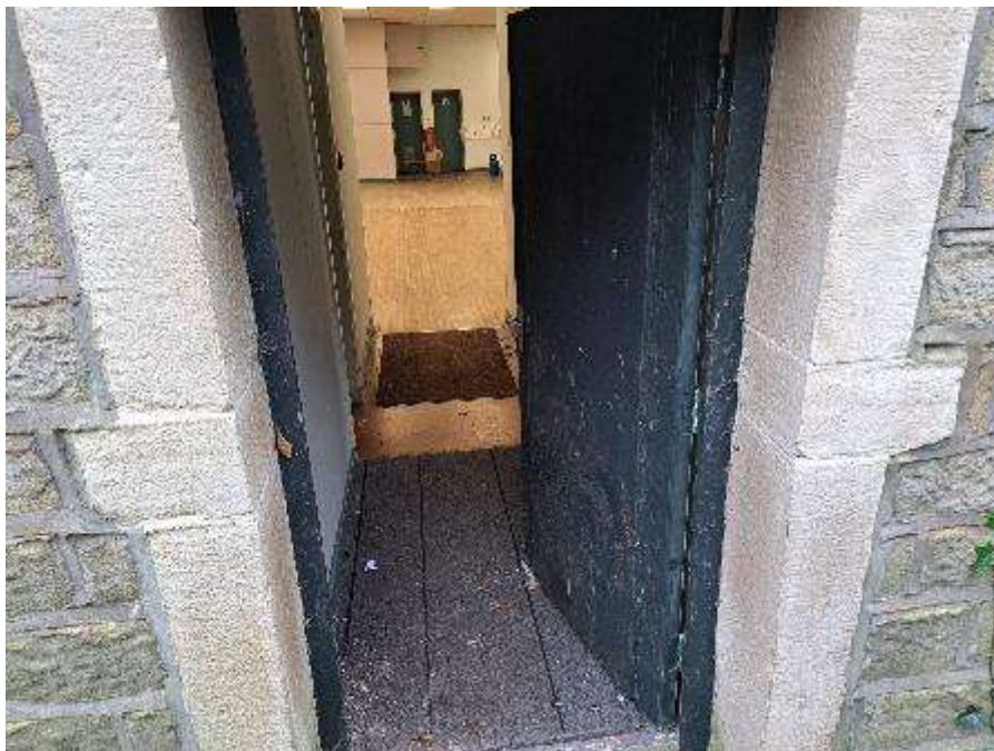
138.Damaged timber door
