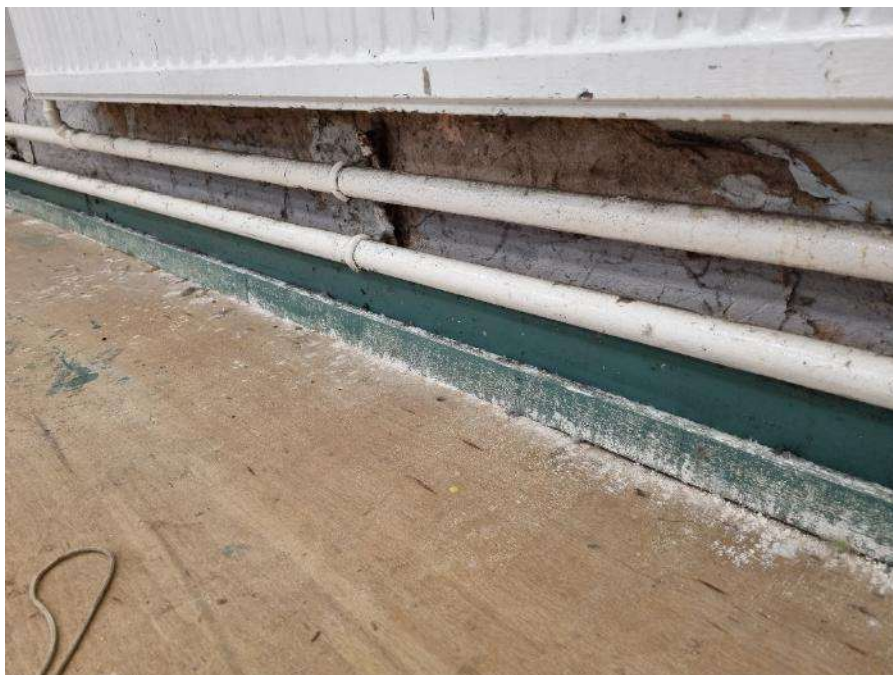
79. View of the defective plaster behind the radiator
