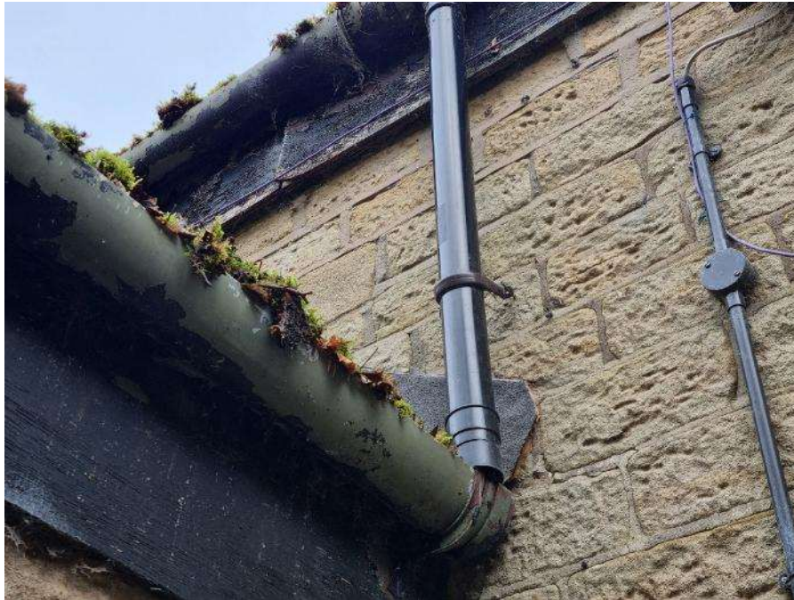
103. Fascias and guttering is in poor condition
