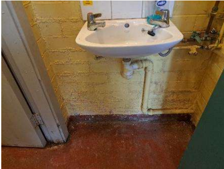
13. Damp present under the Female WC sink
