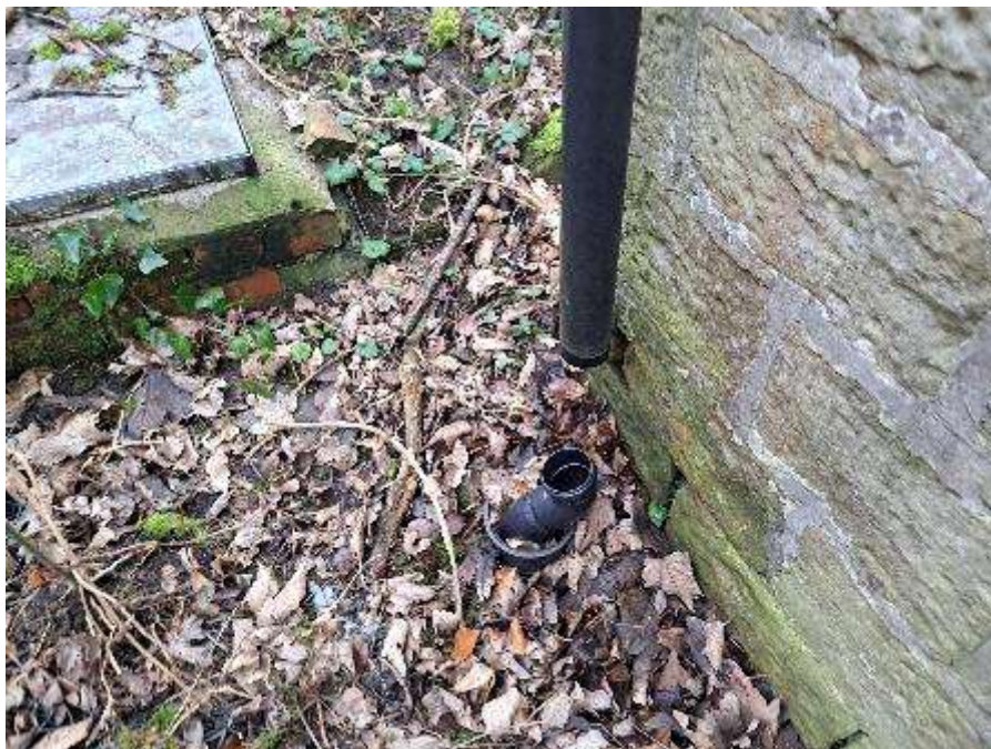
136. Damaged uPVC downpipe
