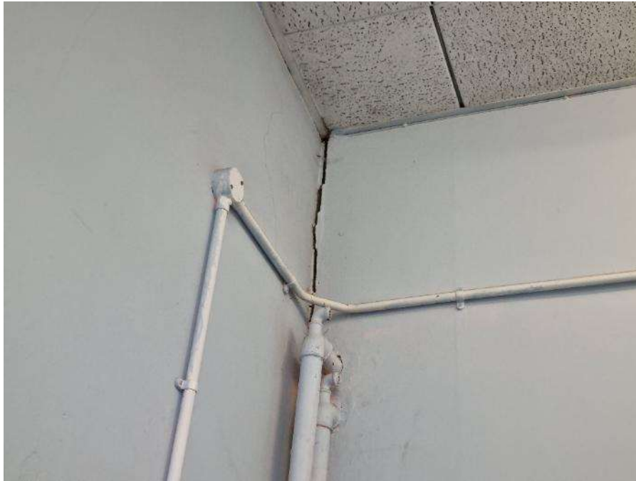
61. Cracking has been noted due to movement in the gable wall
