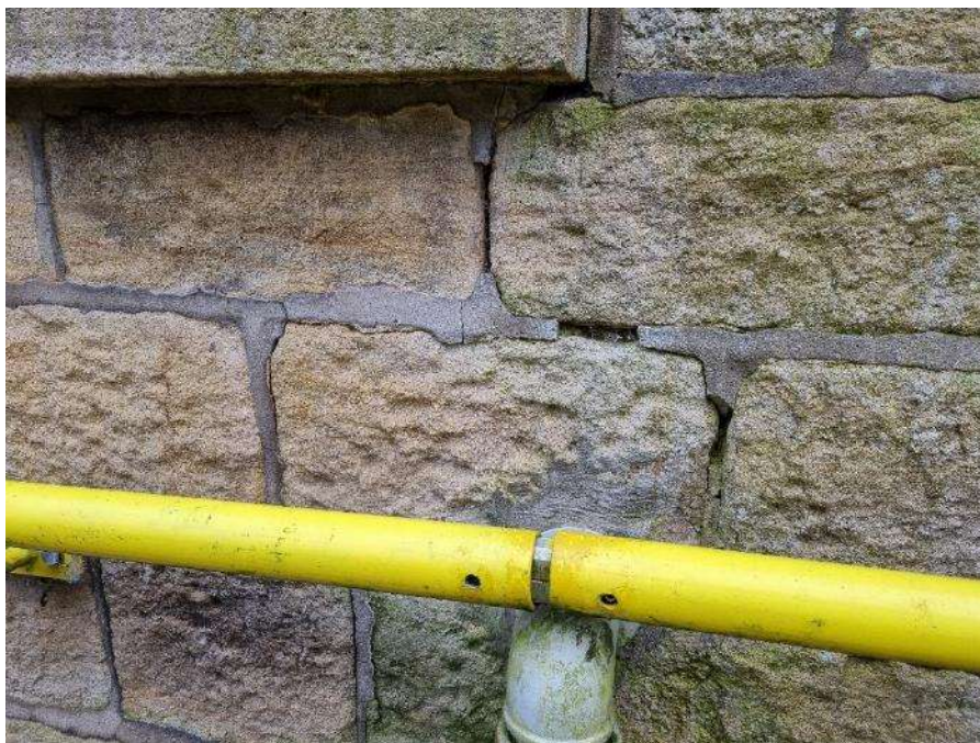
111. Poor condition of the pointing
