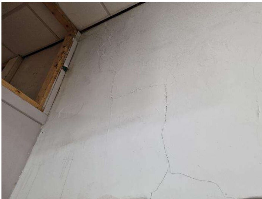
89. Sign of cracking noted to the wall
