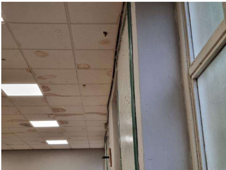
83. Walls are twisted and bulging in various areas
