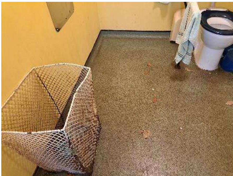
30. Rusted bin and debris
