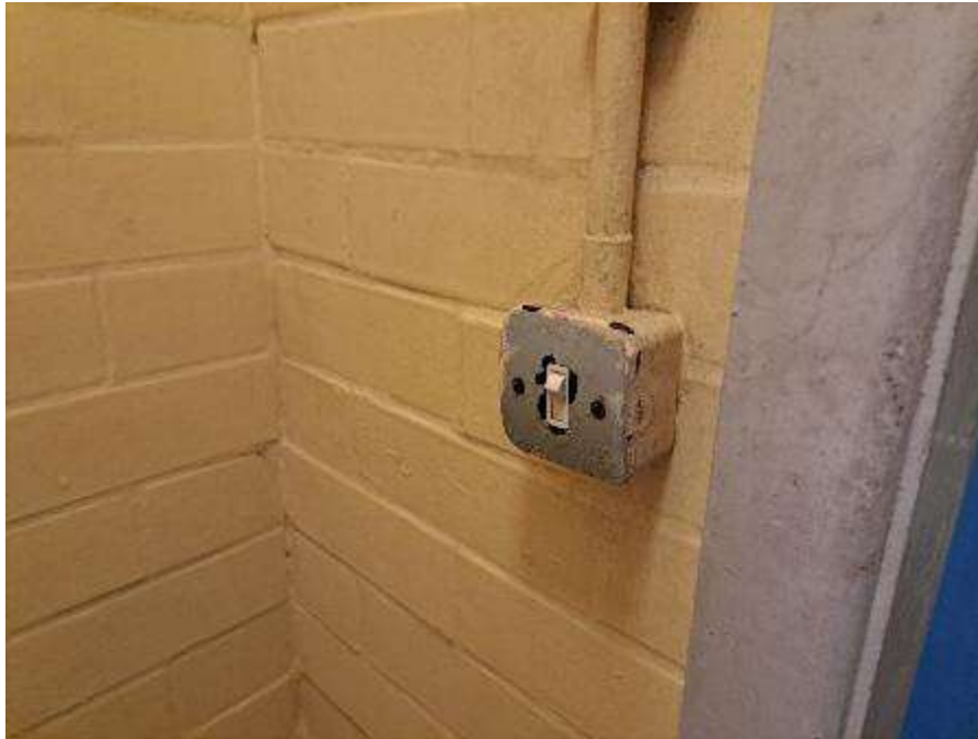
5. Damaged light switch
