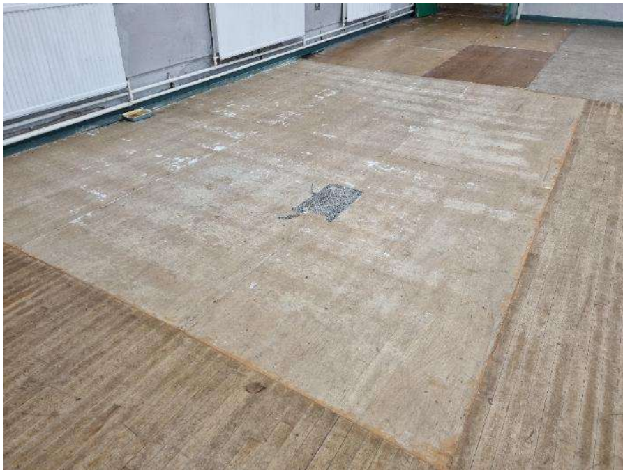
74. Floor is in poor condition, soft underfoot and signs of mycelium
