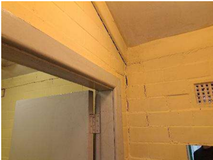
16. Cracking present at high level
