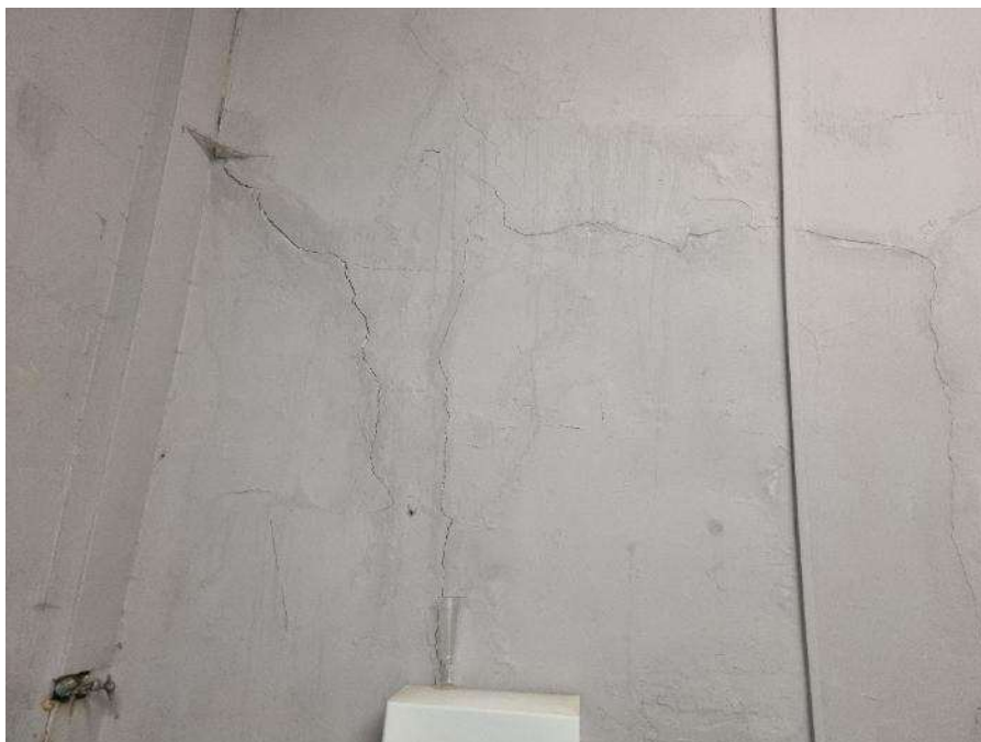
49. Cracking and damp noted to the walls
