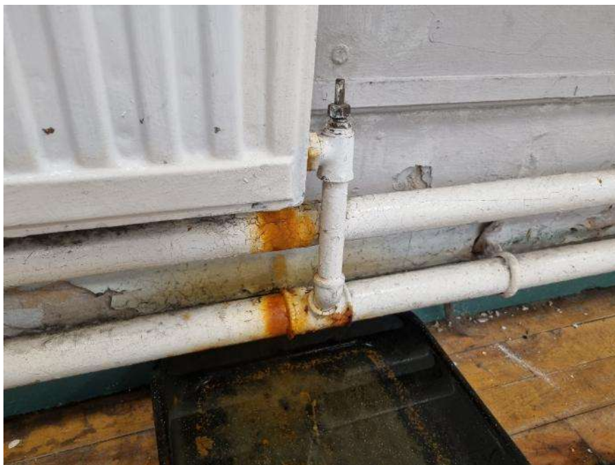
77. Floor is in poor condition due to pipe leaking below the radiator
