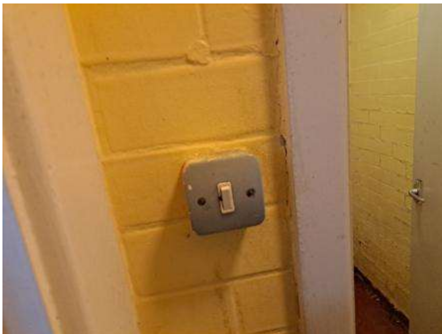
17. Rusted and damaged light switch
