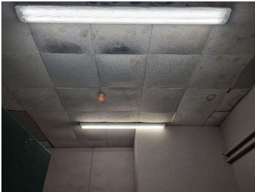
48. Suspended ceiling is in poor condition
