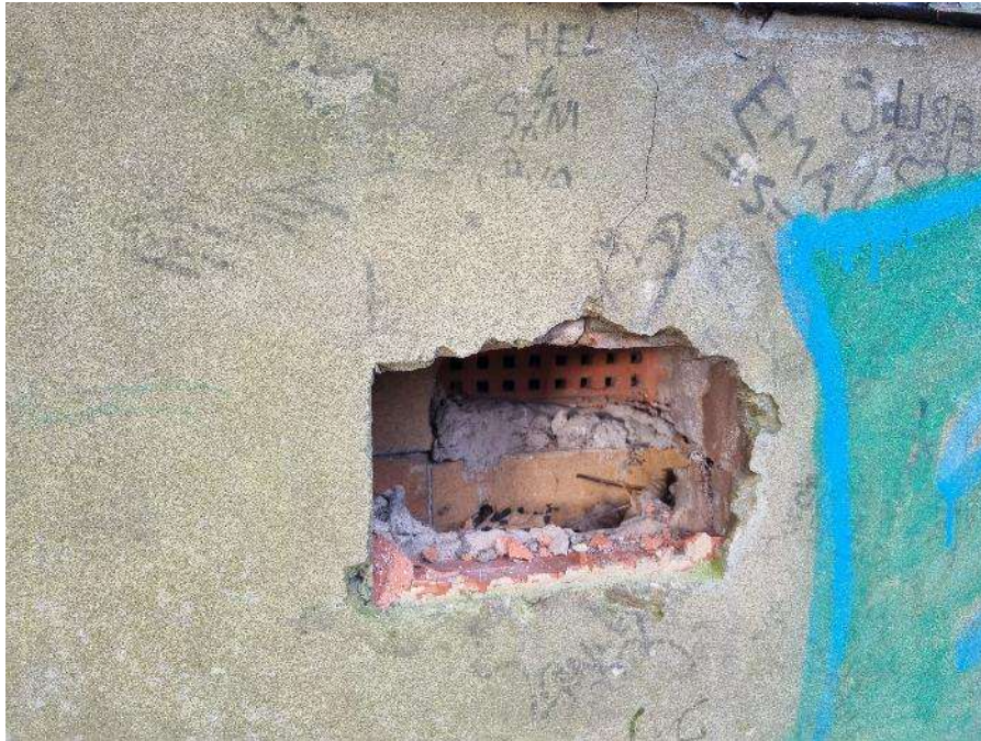
123. Holes within the render
