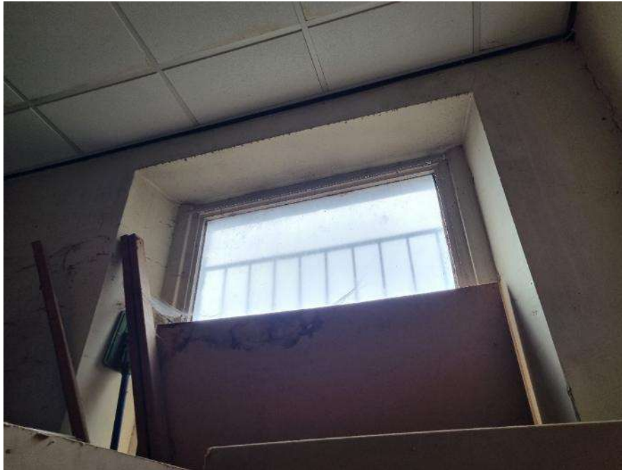
71. Windows are in poor condition.
