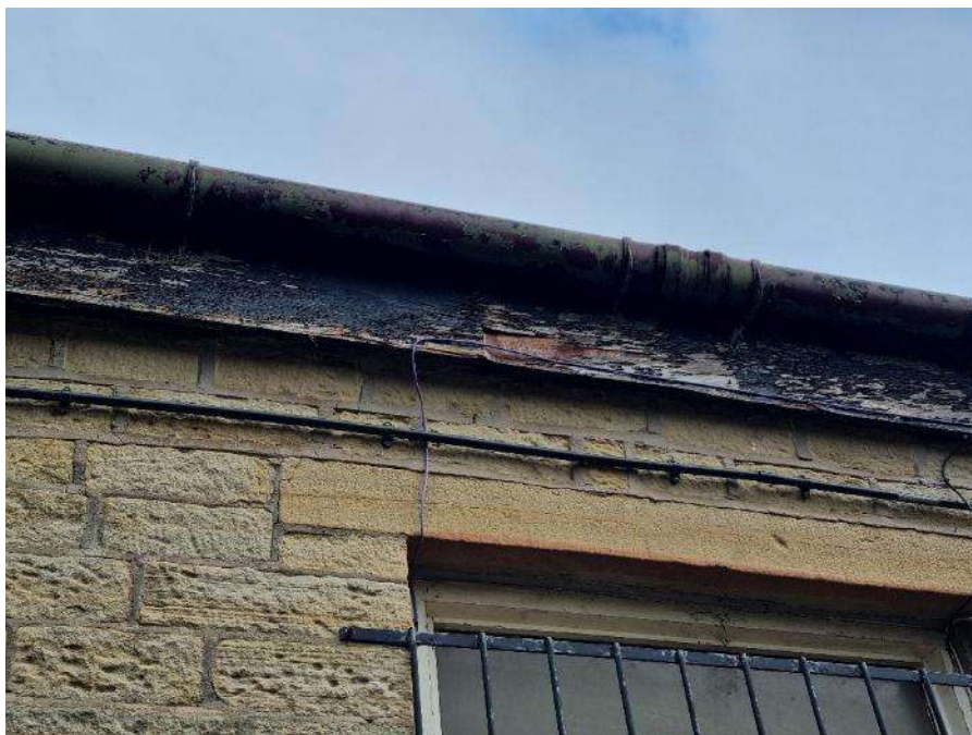
101. Fascias and guttering is in poor condition
