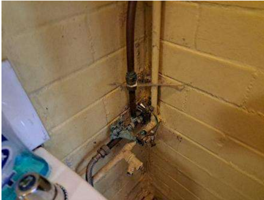
23. Poor decoration to the pipework
