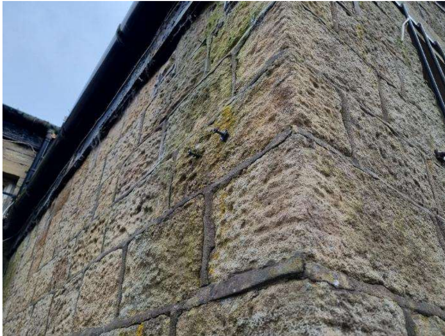
105. Missing downpipe and poor pointing.
