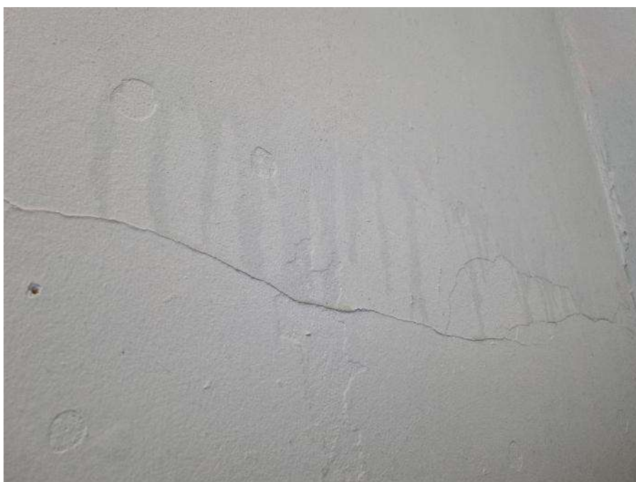
60. Minor hairline cracking noted.
