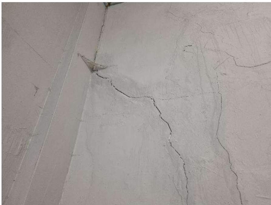
51. Cracking noted to the walls
