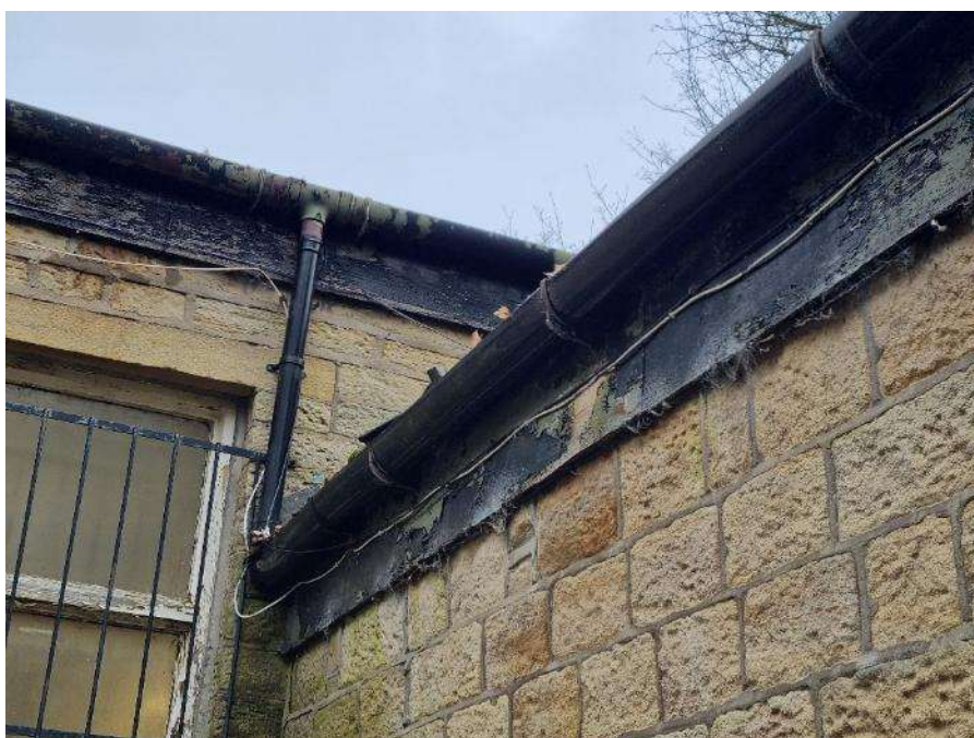
102. Fascias and guttering is in poor condition
