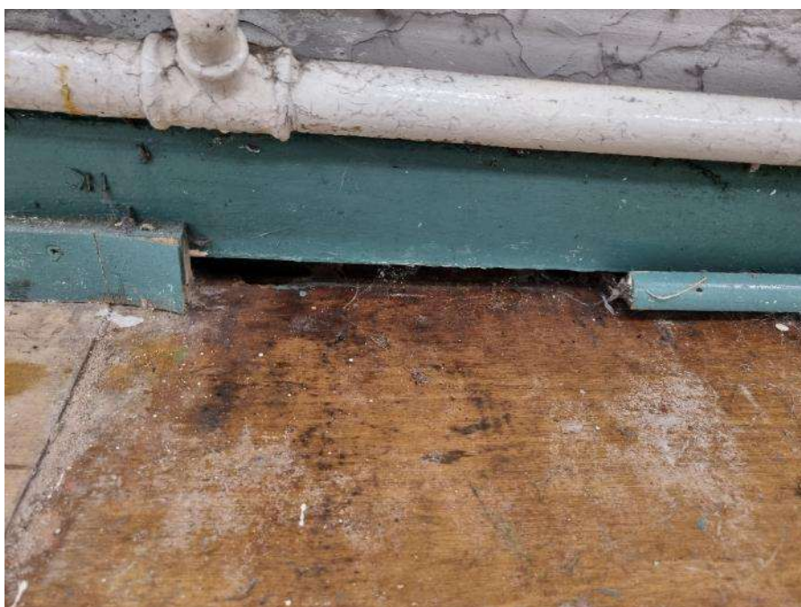
80. The floor in the hall is undulating and missing trim has been noted
