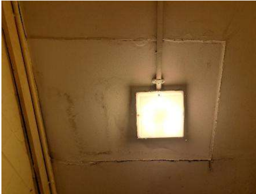
11. Damage to the ceiling decoration with high moisture present
