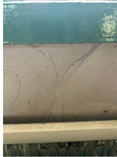
14) , 15) and 16) wall crack under sill and rotten sill and windows (B)
