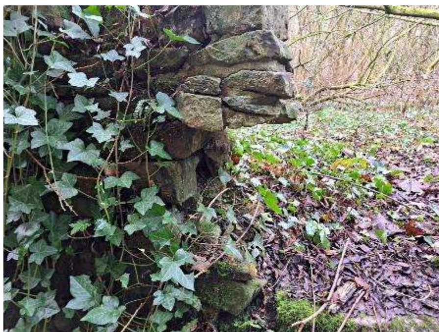
142.Damage to perimeter/boundary wall
