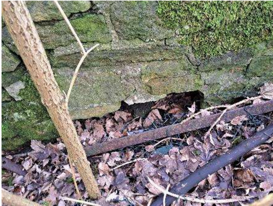
135. Damaged retaining wall
