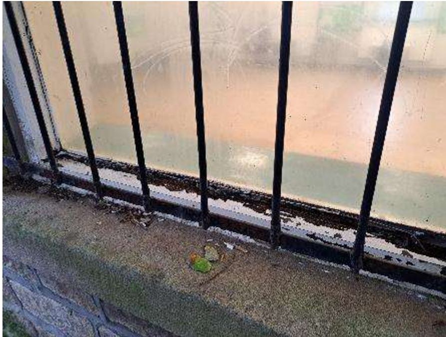
133. Damaged windows and rusted bars
