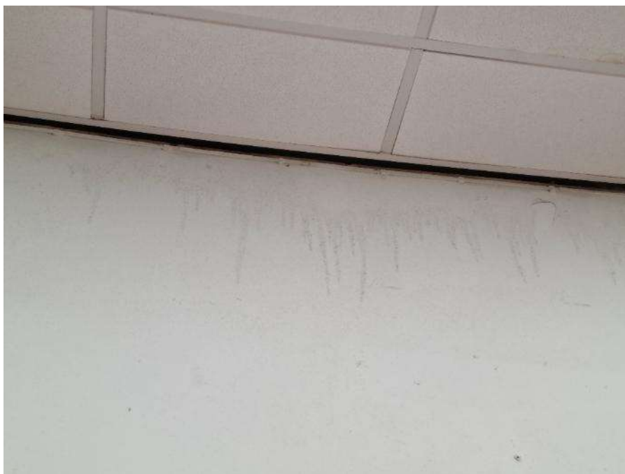
86. Signs of water ingress noted towards ceiling
