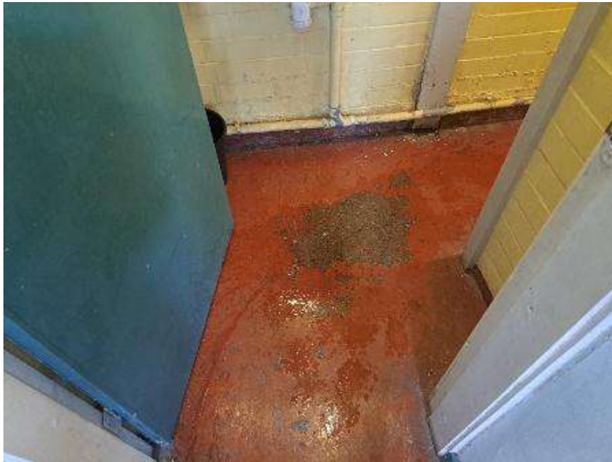
1. Damage to the concrete floor
