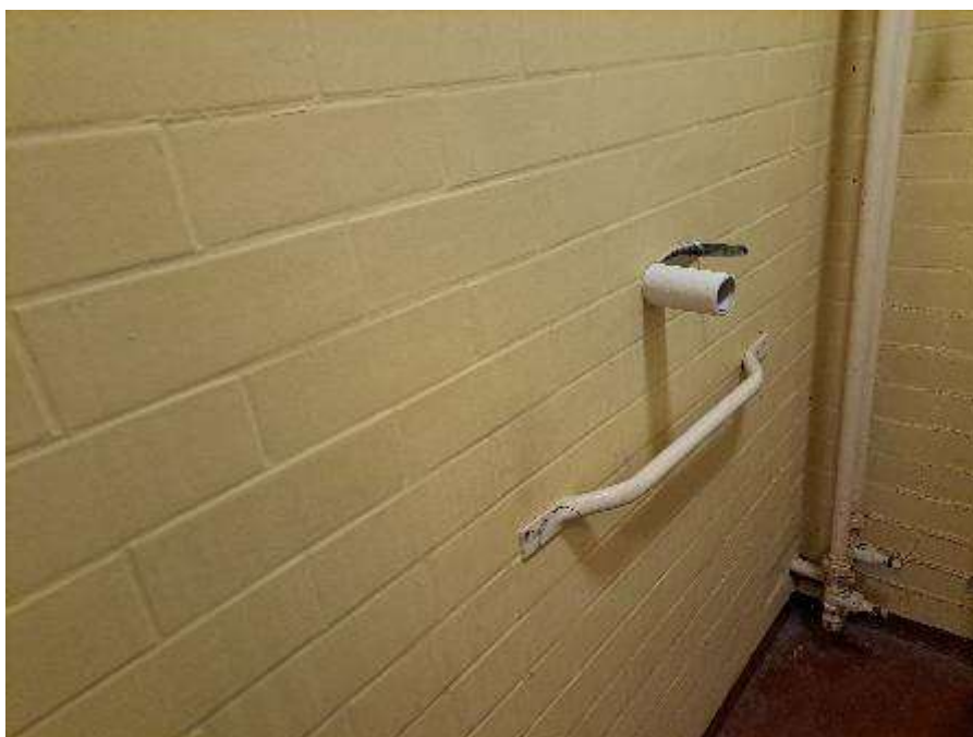
22. Damage to the metal handrail
