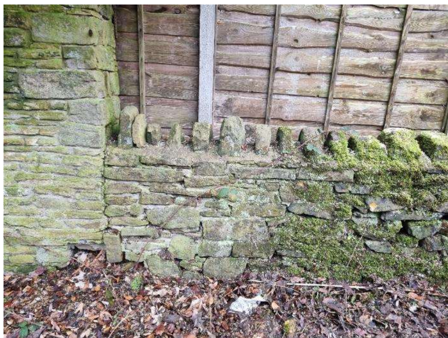
115. Boundary Wall is in poor condition
