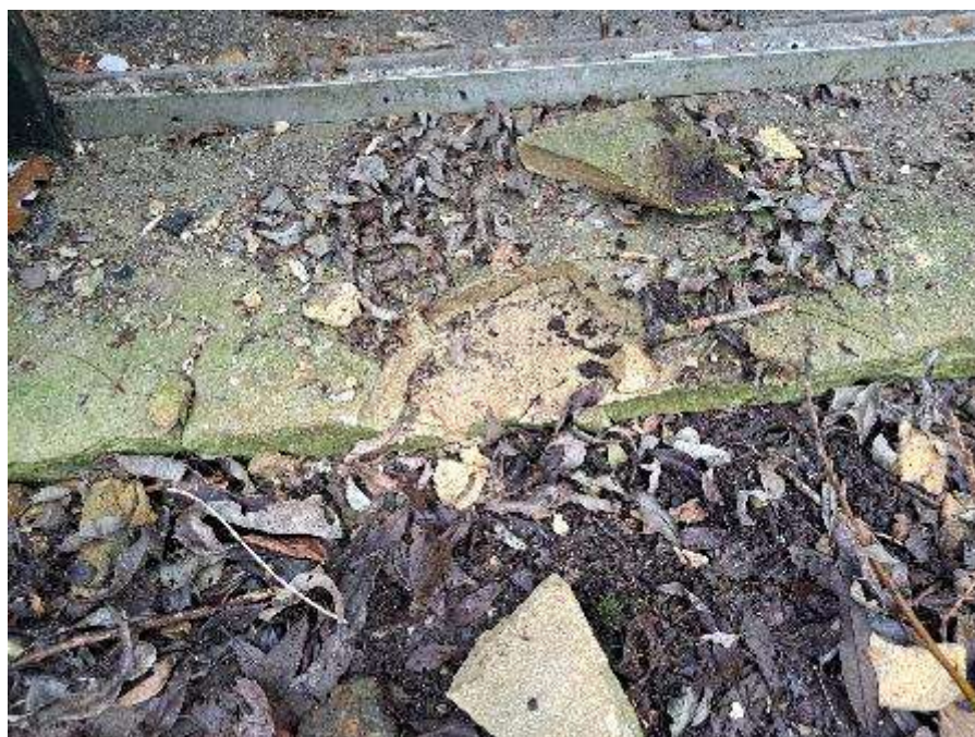
141.View of damaged step
