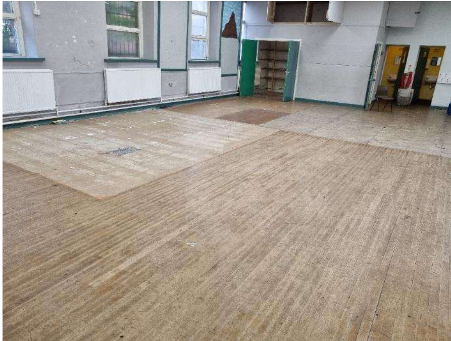
73. View of damaged floor within the hall.
