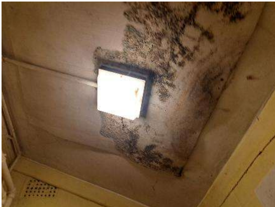
24. Damage to the ceiling due to the water ingress
