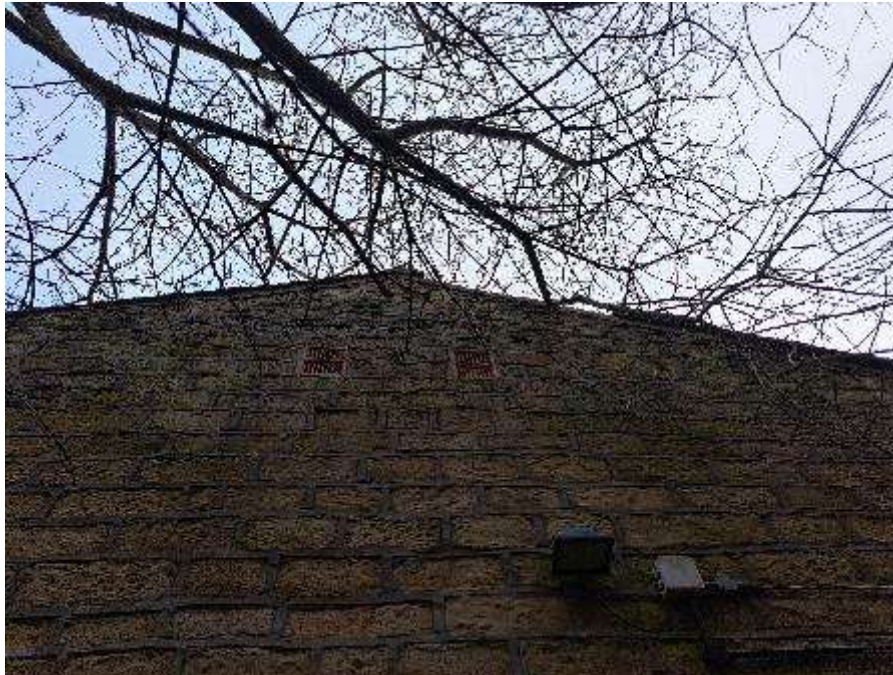
139. Damaged roof due to tree
