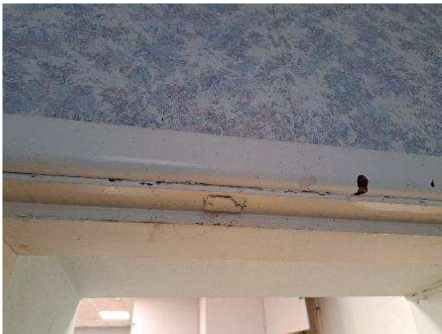
37. Damaged timber architrave
