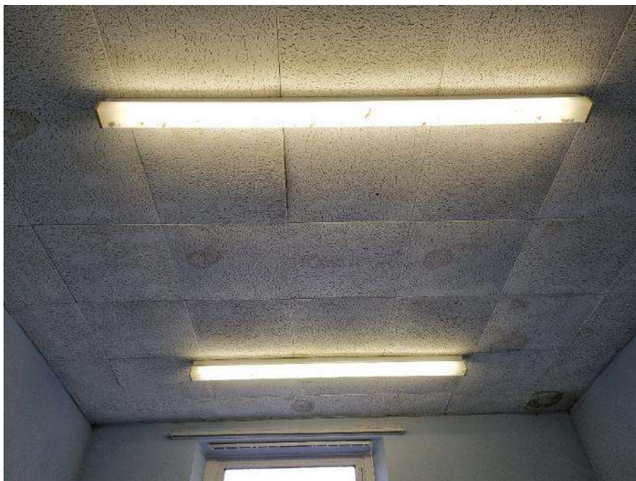
59. Ceiling is in poor condition
