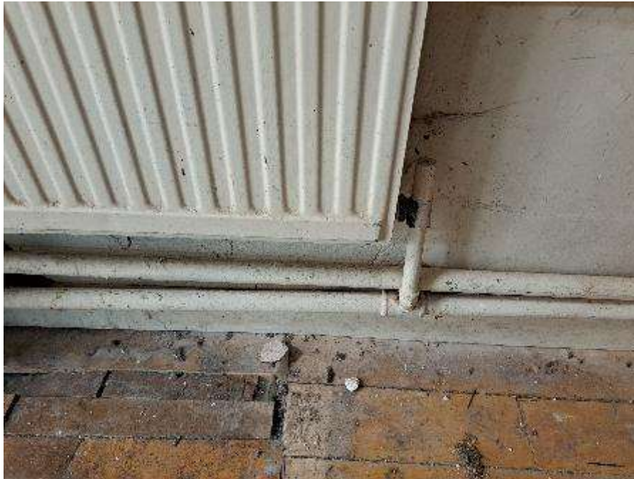
45. View of damaged floor
