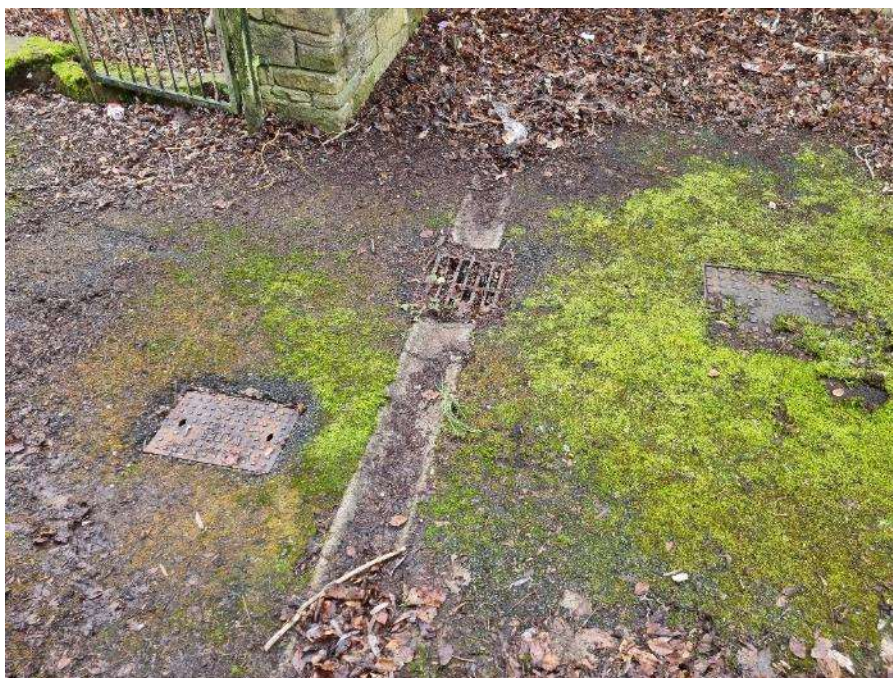
112. Moss and debris filled floor.
