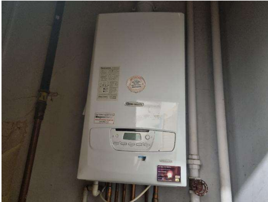
53. General view of the boiler
