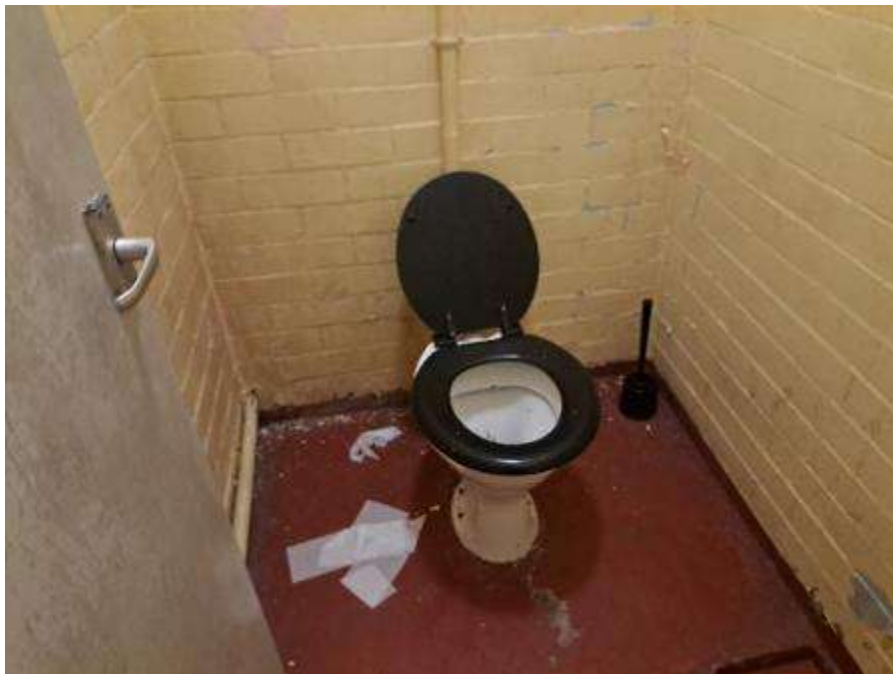
6. Damaged and aged WC
