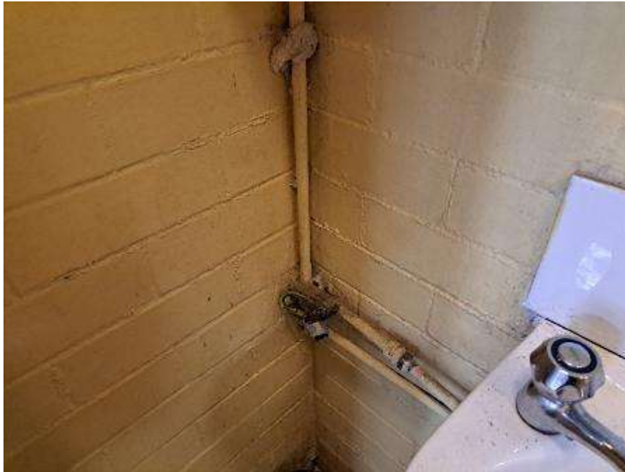
3. View of poor decoration to the pipework
