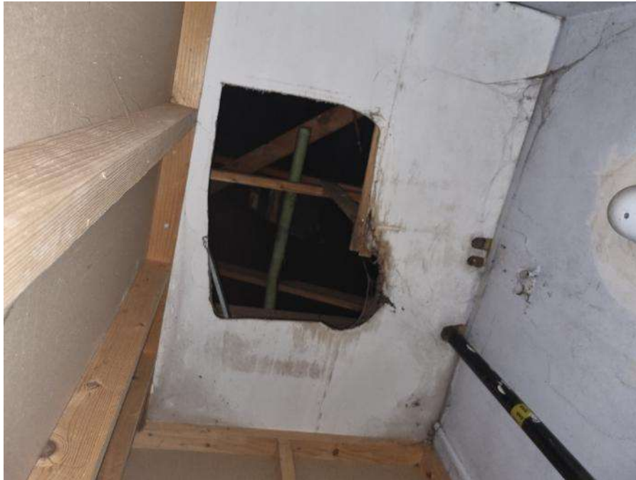
55. Poor condition of the ceiling
