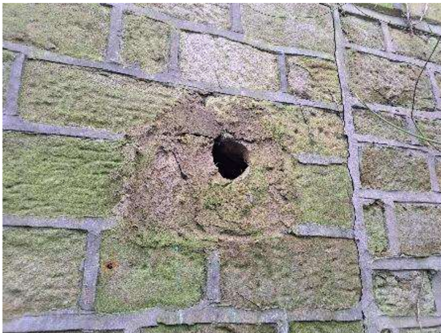
128. Penetration to the wall
