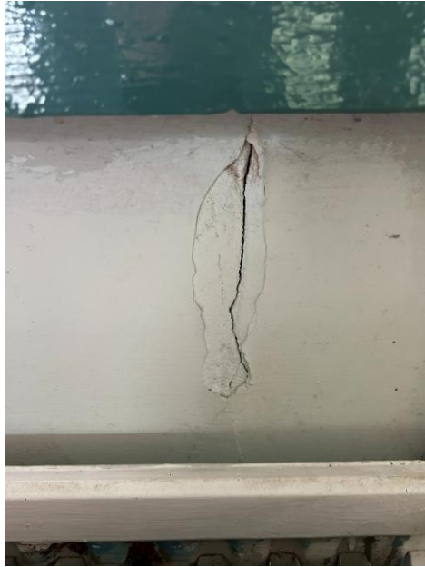
8) Small structural crack below sill (C)
