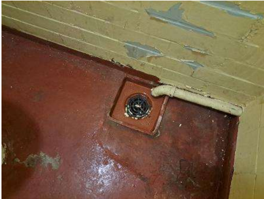
7. View of unsanitary drain and poor decoration
