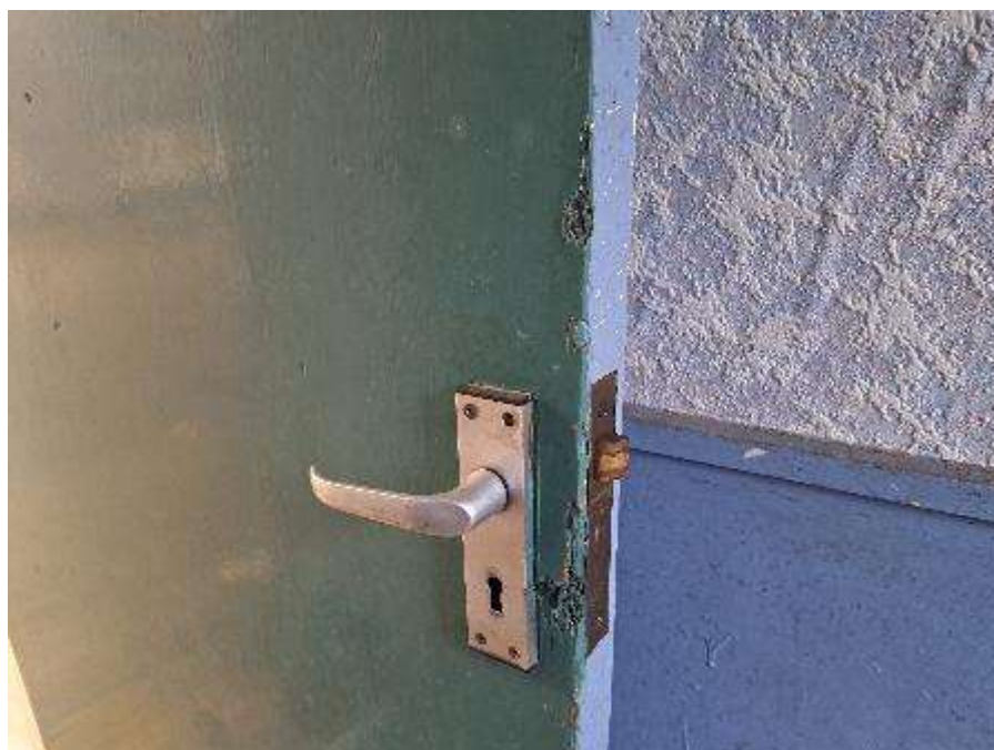
36. Damaged timber door
