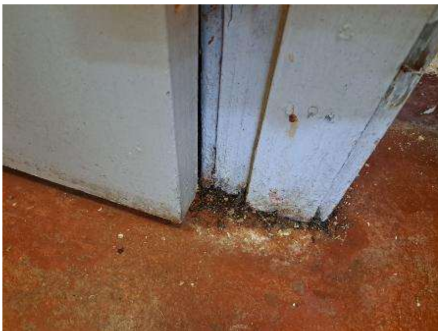
18. Poor decoration/damaged architrave
