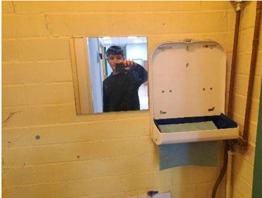
15. Damaged hand towel unit
