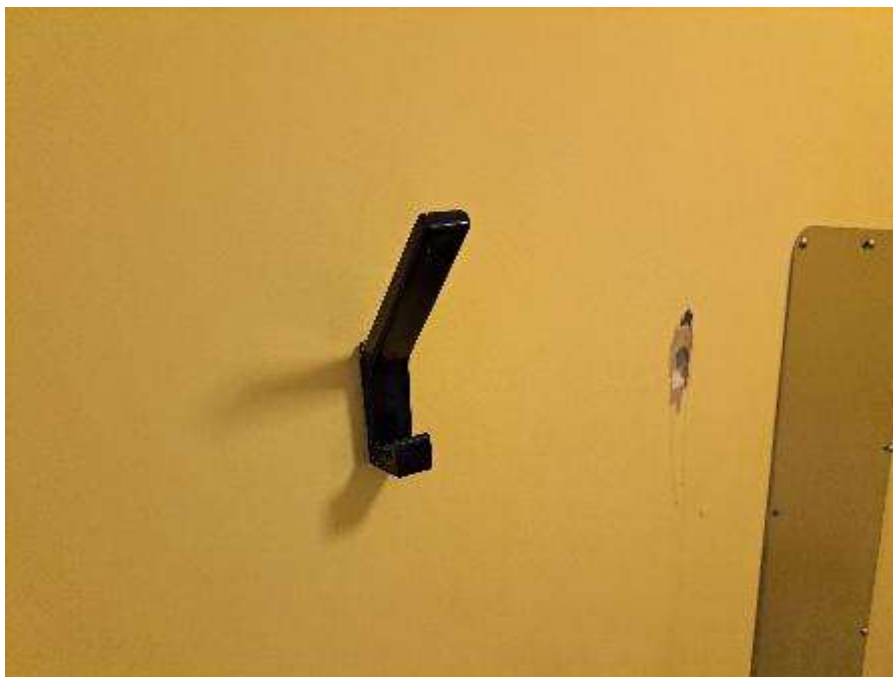
29. Damage from a previous coat hook
