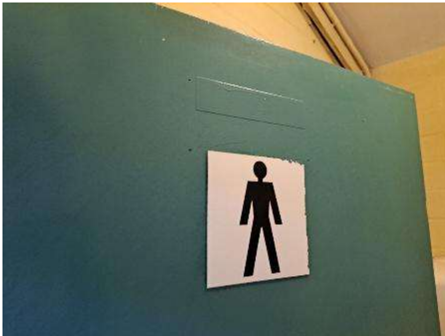
12. Penetration holes to the timber door
