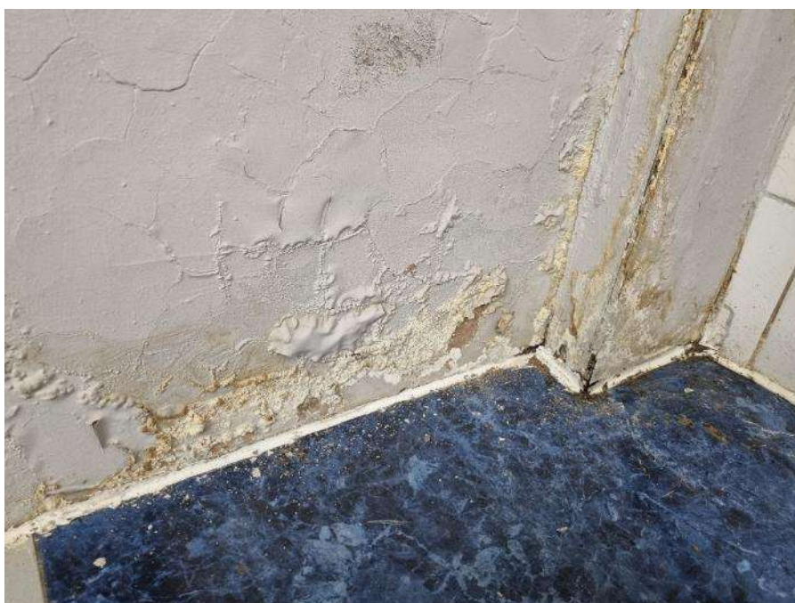
50. Extensive damp noted to the walls.
