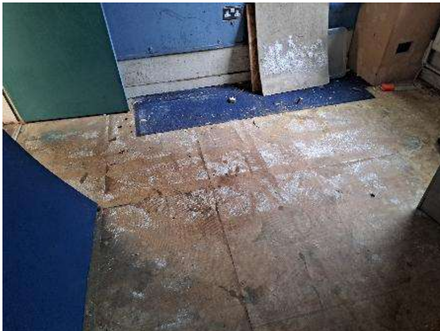
34. Damaged floor covering and fungi / mycelium spores
