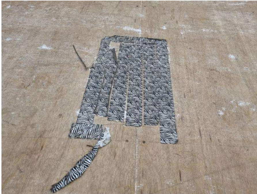
75. Floor is in poor condition, soft underfoot and signs of mycelium
