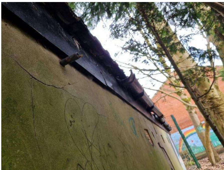
126. Damage to the render and guttering.
