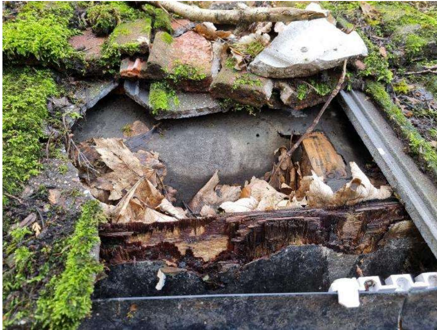
95. View of damaged roof
