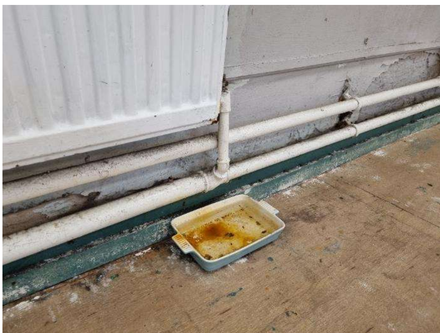
78. Floor is in poor condition due to pipe leaking below the radiator
