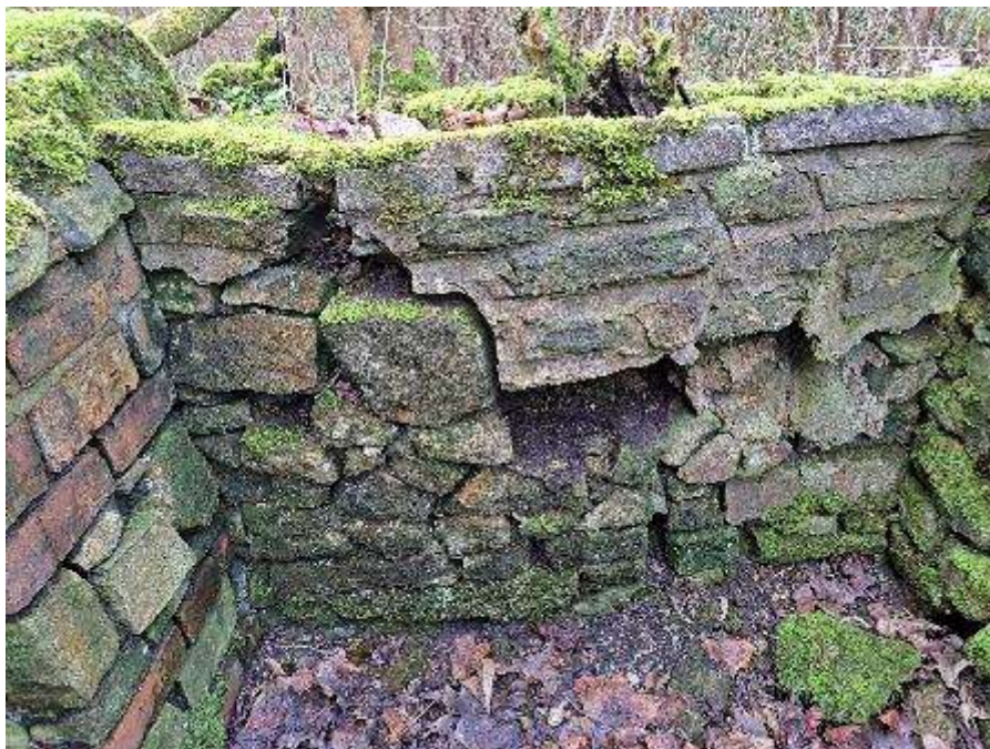
134. Damaged retaining wall
