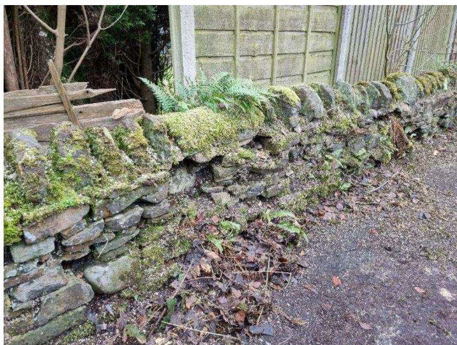
116. Boundary Wall is in poor condition
