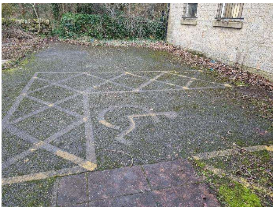
114. Disabled parking bay is in poor condition
