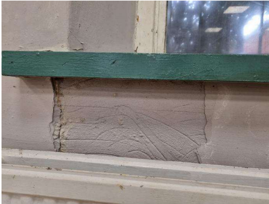
81. Defective plaster noted to below the window
