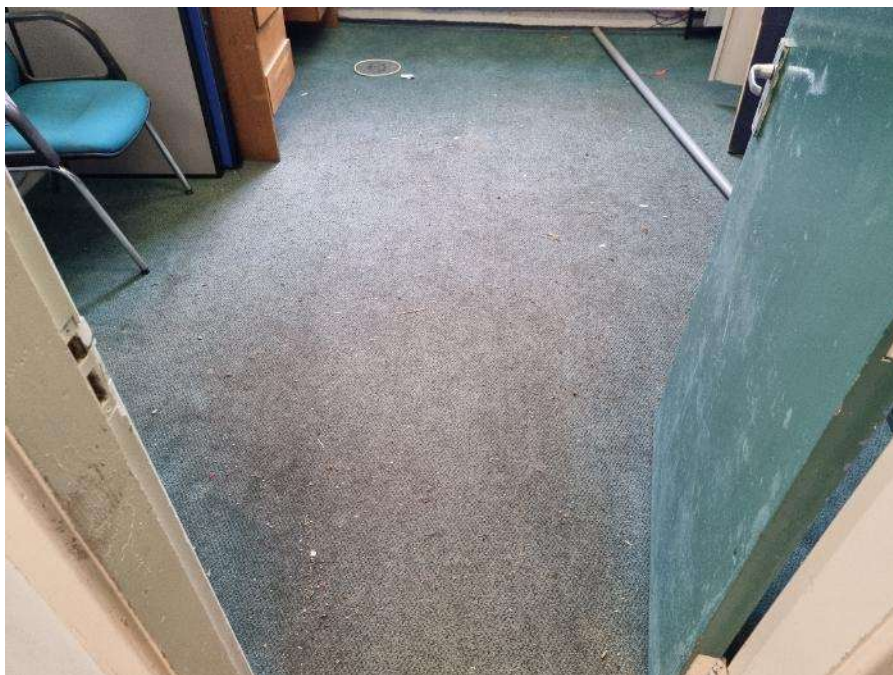
57. Carpet is in poor condition to the office.
