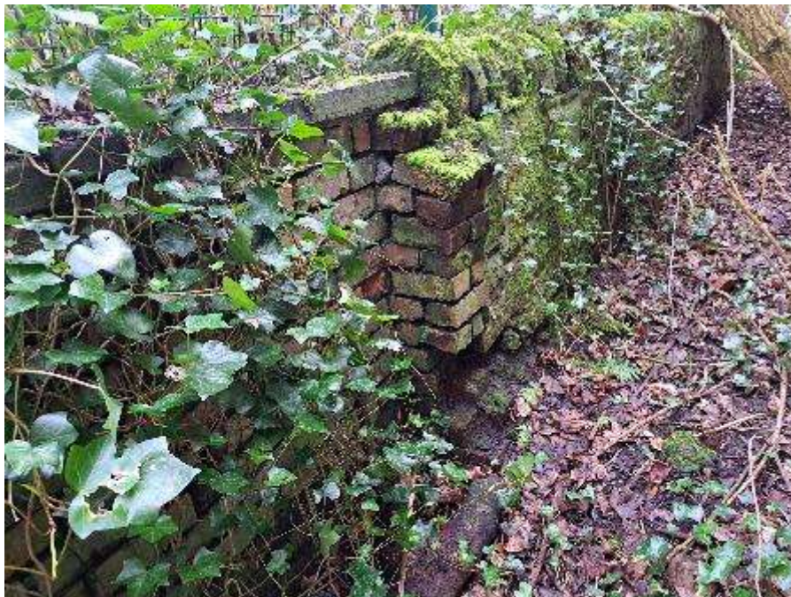
130.View of damaged wall
