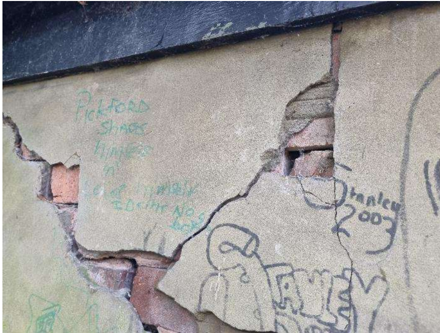
125. Damage to the render
