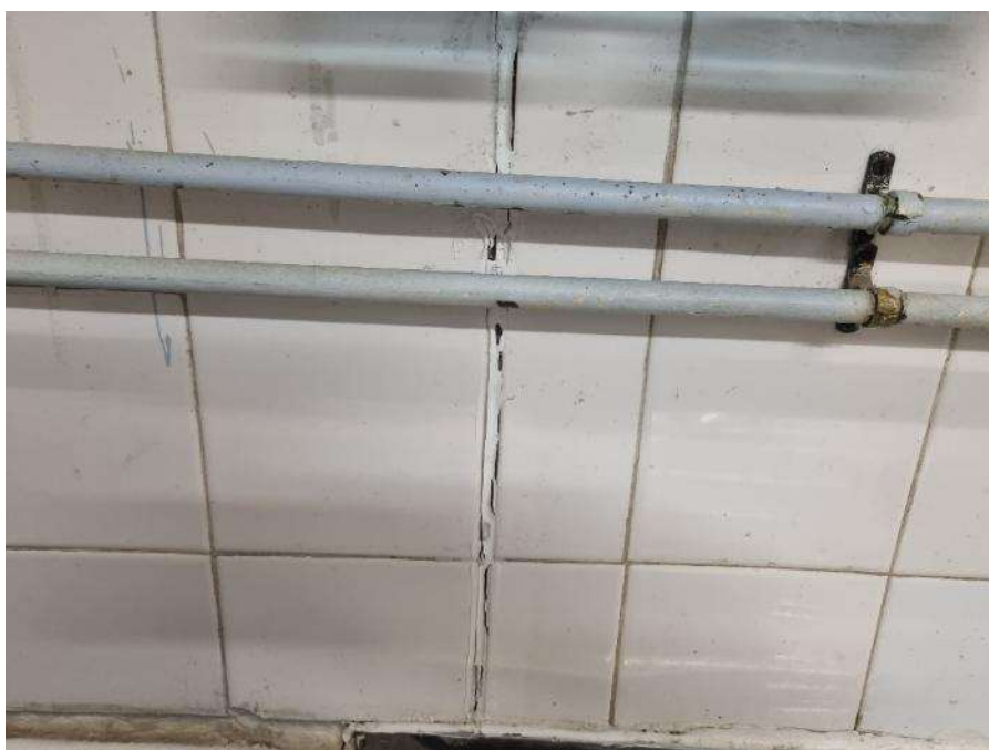
52. Cracking noted to the walls
