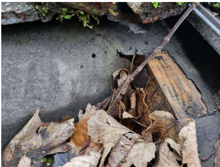
96. View of damaged roof covering
