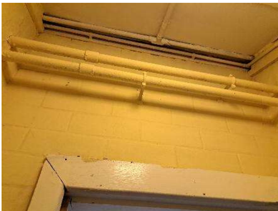
10. Poor decoration to pipework
