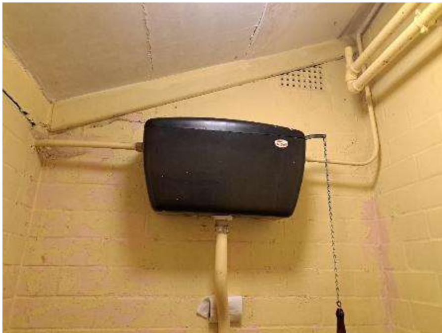
8. View of blocked air vent and aged WC
