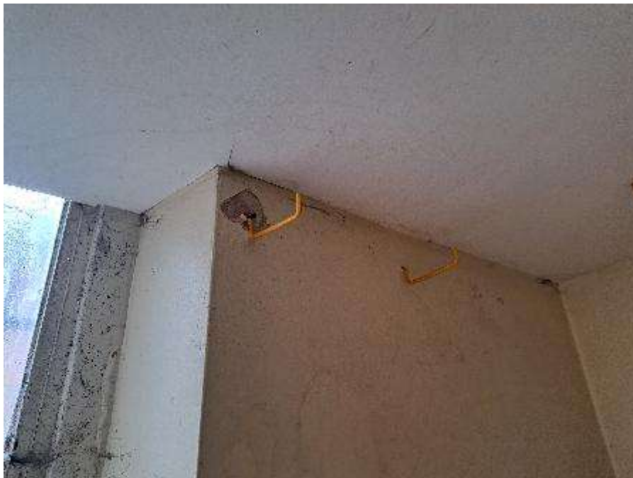
42. Damaged wall due to fixings
