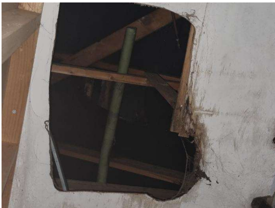
56. Roof timbers are in fair condition and the felt is defective.
