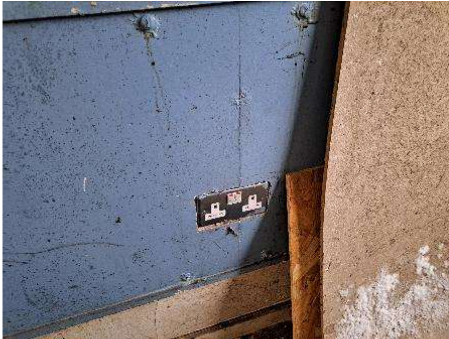
41. Damaged wall and plug socket
