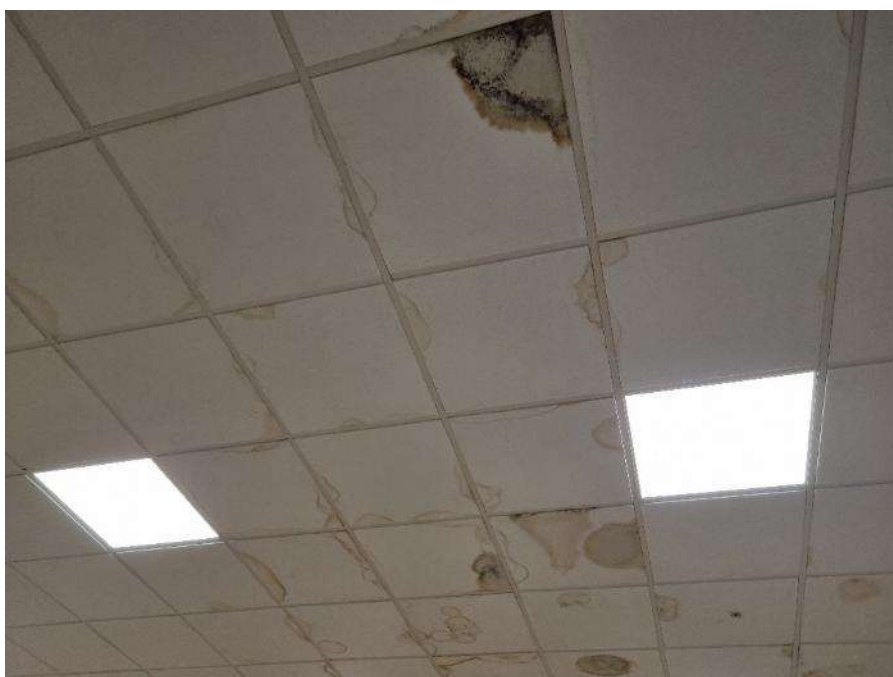
84. Ceiling is in poor condition
