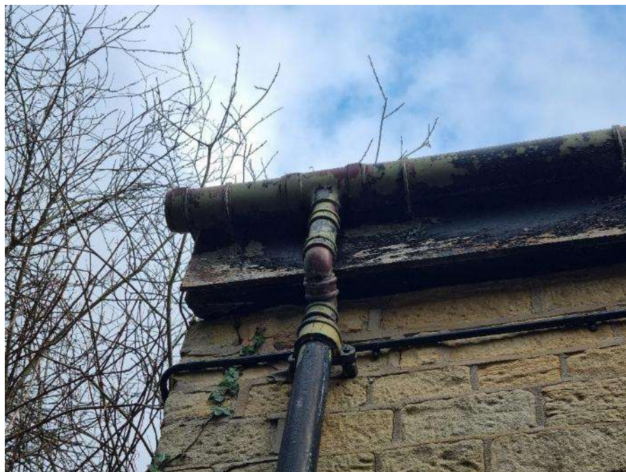
99. Poor condition of fascia's and rainwater
