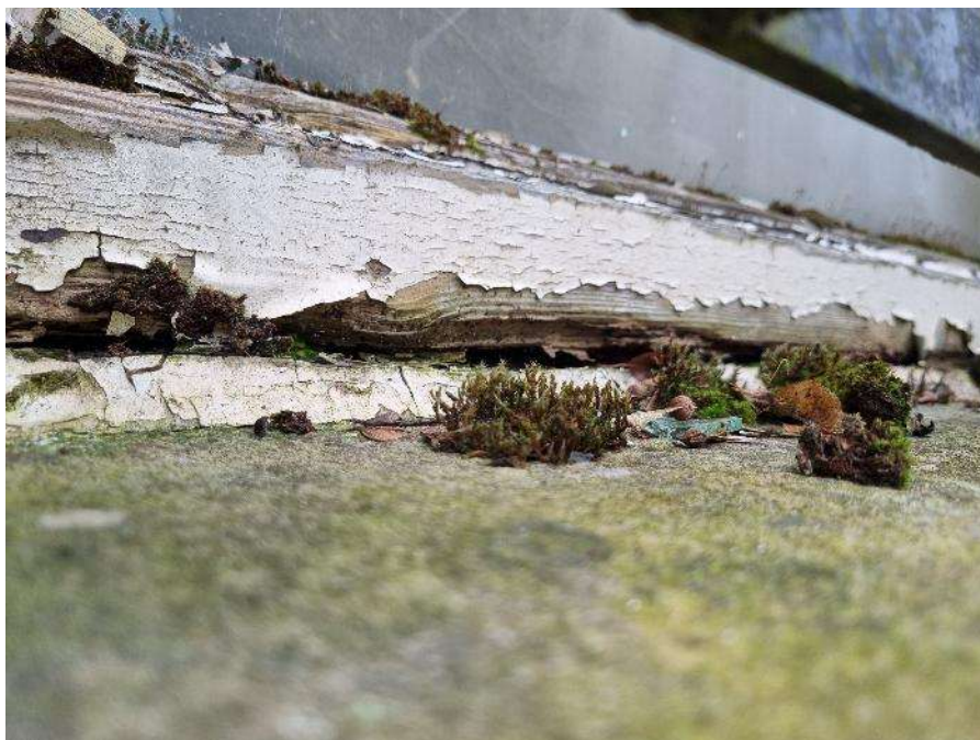
109. Window is in poor condition
