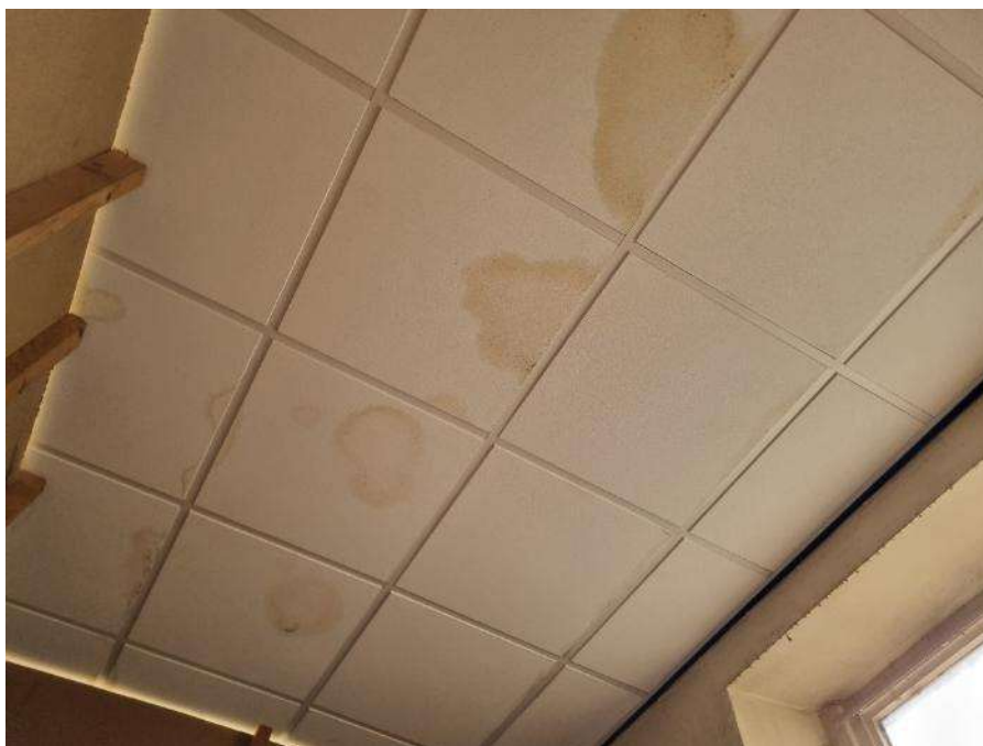
70. Ceiling is in poor condition
