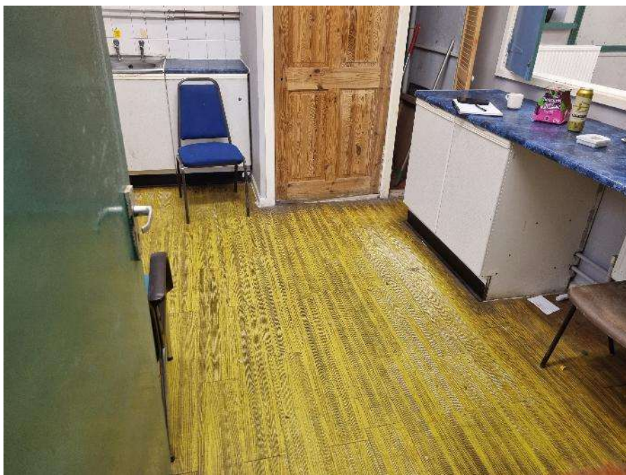
46. View of floor which is nearing the end of its serviceable life.
