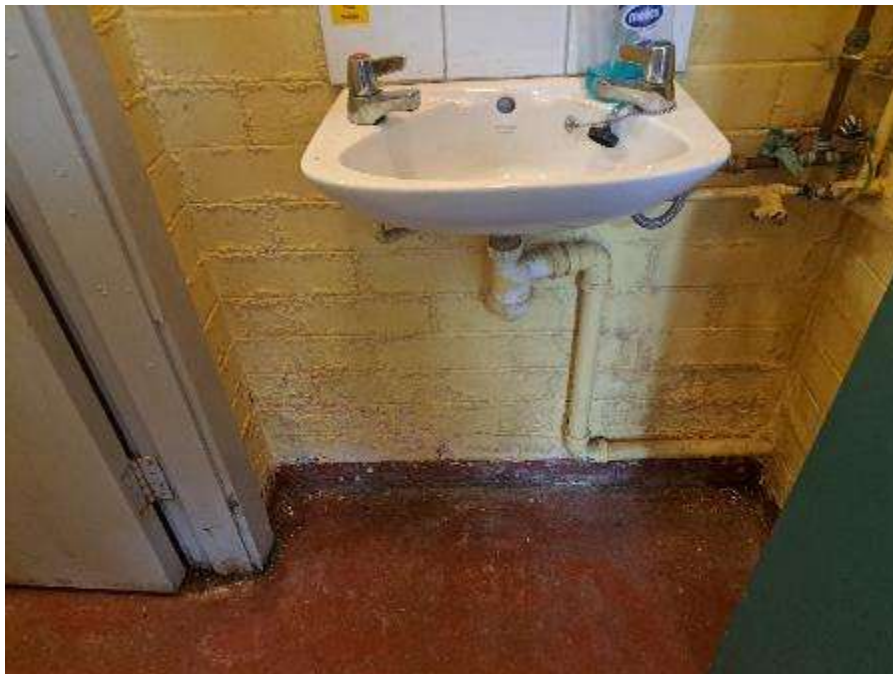
14. Dirty and aged sink unit
