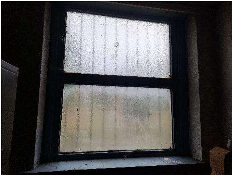
40. View of damaged timber window
