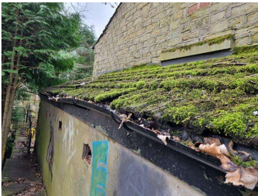
120. Lean to roof is in poor condition
