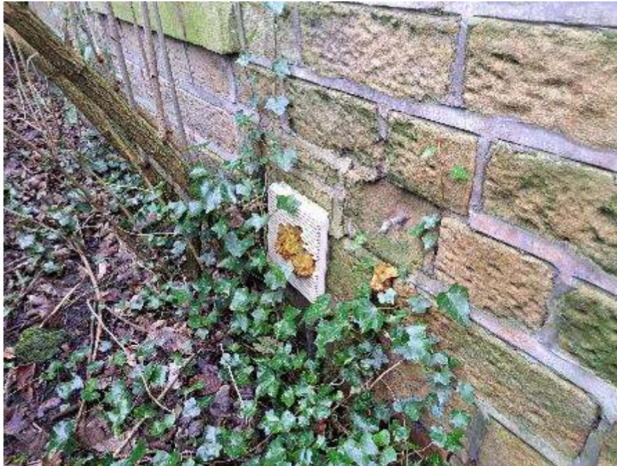
129.View of damaged vent
