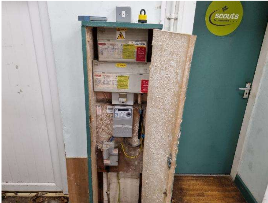
87. View of the main incoming electrics
