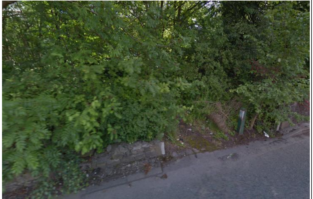
Figure 4: Photograph showing the gap on the wall at approximate NGR SJ9517998124
